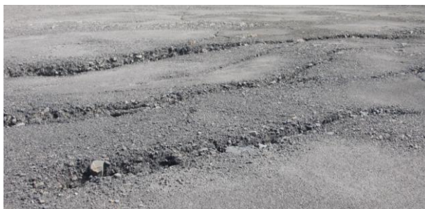
Figure 2: Cracks on the dump surface
